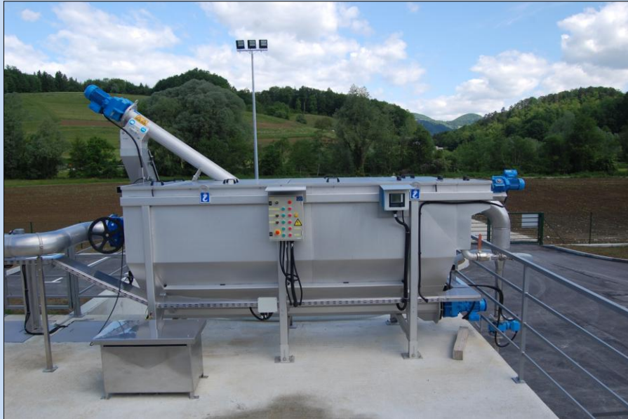
MECHANICAL TREATMENT PLANT – SAND & GREASE TRAP
