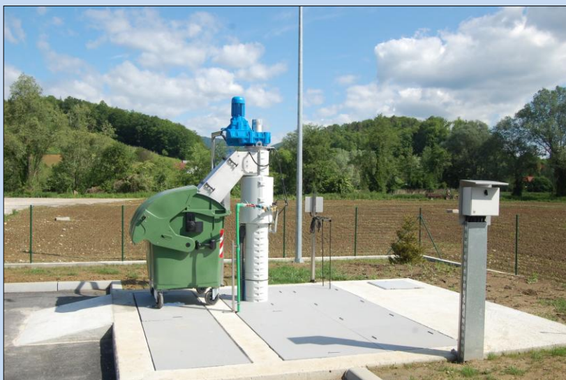
INLET PUMPING STATION WITH FINE SCREEN
