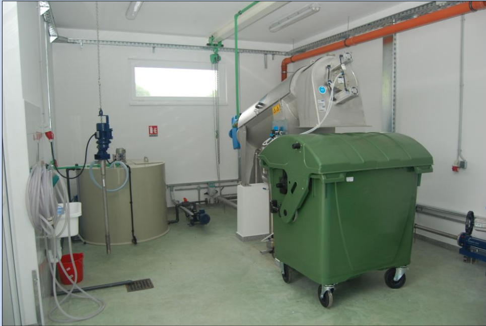
DEHIDRATION PLANT WITH FILTER PRESS
