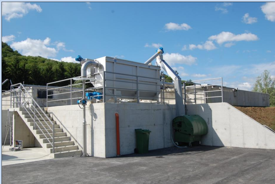
EQUILIZATION TANK WITH MECHANICAL TREATMENT PLANT
